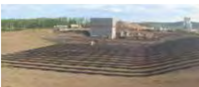
Dry float-sink installation
